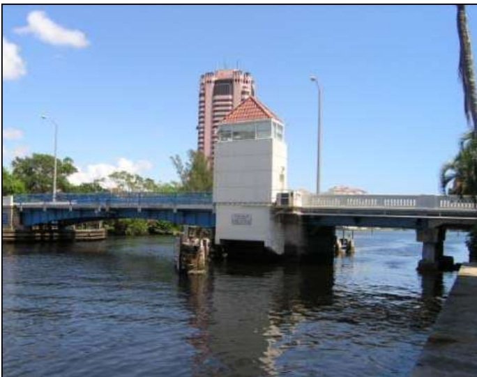
Photo 5-74. Clarence Geist Memorial Bridge/Camino Real Bridge/Boca Raton Club Bridge, Palm Beach County (No. 934408)
